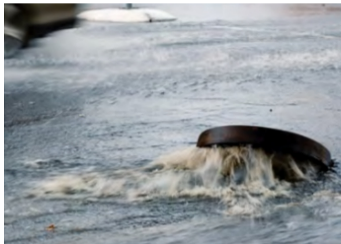
Fig15. Over Flow of the Sewage system
