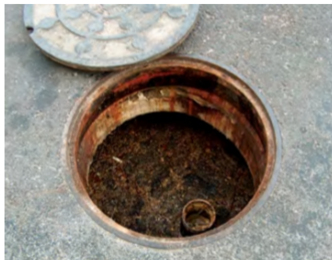
Fig16. Clogged Manhole of the Sewage system
