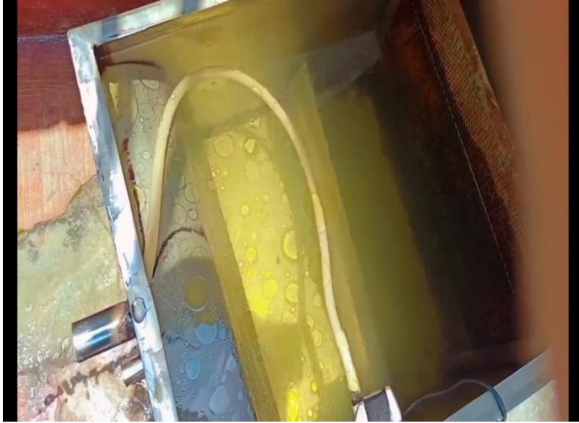
Figure 26 – Outlet of the grease trap with the pump connected to upper outlet.
