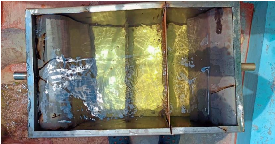
Figure 22 – grease trap with a capacity of 60 liters.
