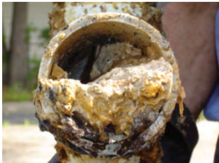
Fig14. Clogged Sewage Pipe Due to the heavy oil.
