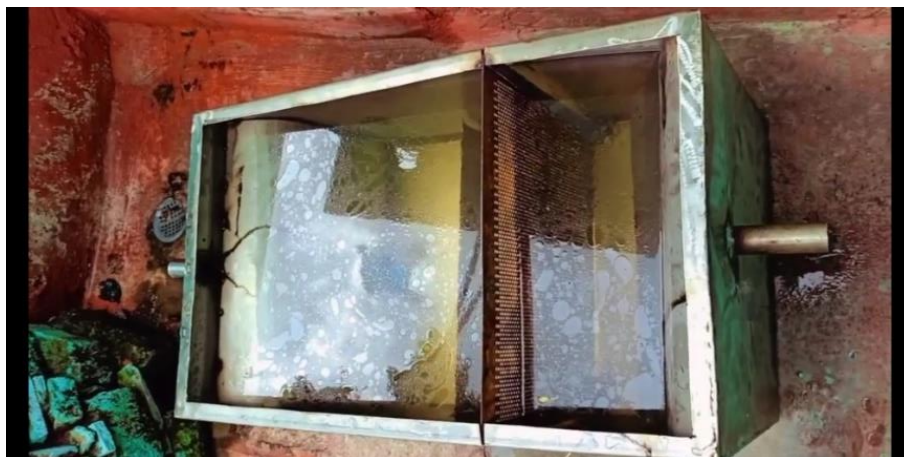
Figure 25 –The grease trap of filled with a mixture of FOG and water.
