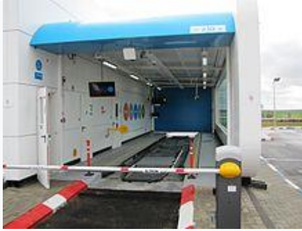
Fig:2.3 A Better Place battery switching station in Israel
